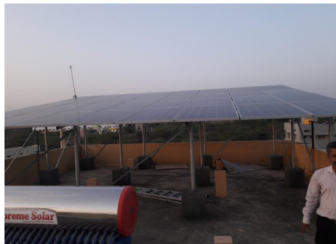
Fig 4. Actual onsite of 8KW solar roof top PV modules at Avaragere, Davangere city
