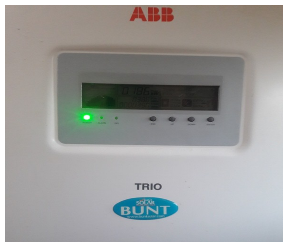
Fig 5. Actual onsite 8KVA solar grid inverter at Avaragere, Davangere city
