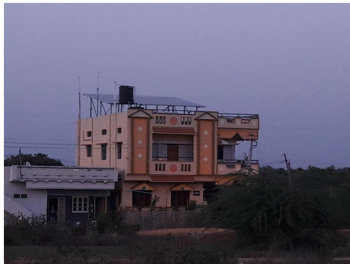
Fig 3. Actual onsite of 8KW solar roof top plant at Avaragere, Davangere city
