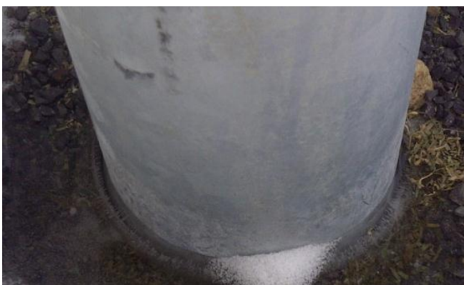
Figure 2. The uplift movement of the pile foundation can be seen at the base of the pile.
