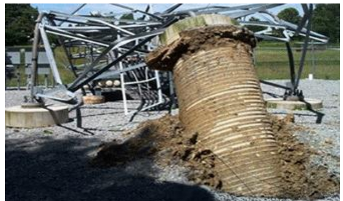
Figure 1: Frost uplift failing a tower foundation.
