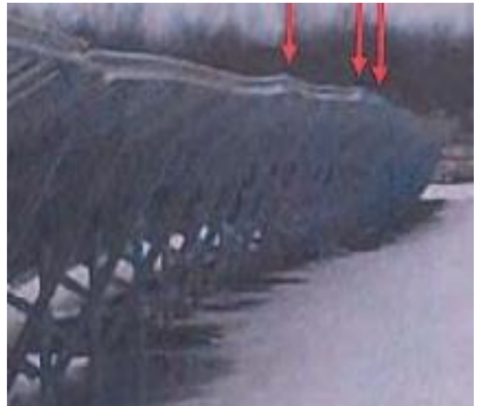
Figure 3. Piles affected by frost showing deformation of the racking with red arrows.
