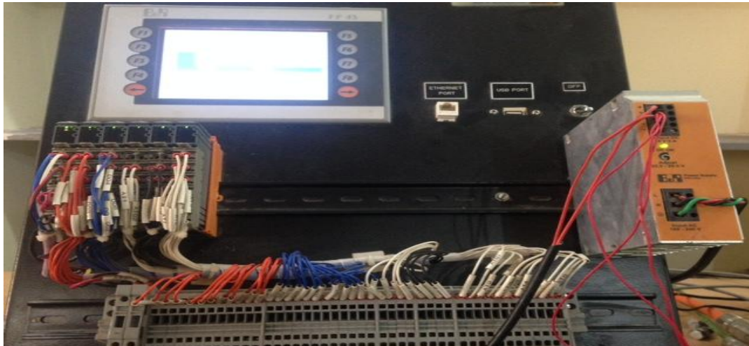
Figure 10: PLC with HMI
