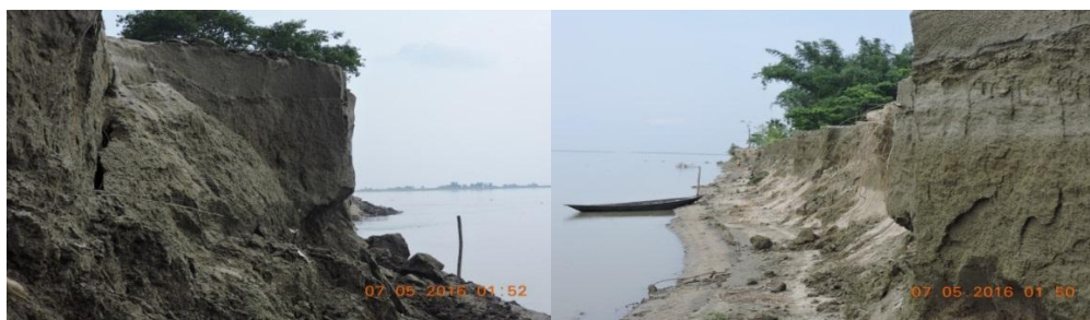
Image: Bank erosion at Boralimari.
