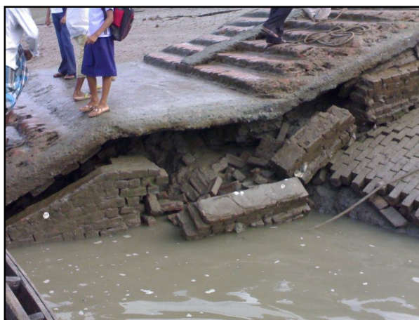
Plate 1: Erosion due to undercurrents at the ferry ghat near Basanti Bazaar, 2008
