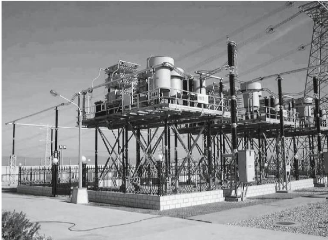
Fig.2 Thyristor-controlled series capacitor (TCSC) installation
