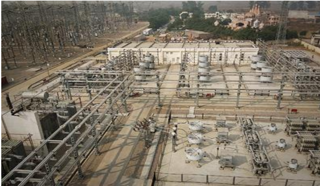
Fig.4 Static VAr compensator at Ludhiana (- 400 MVar / + 600 MVar)
