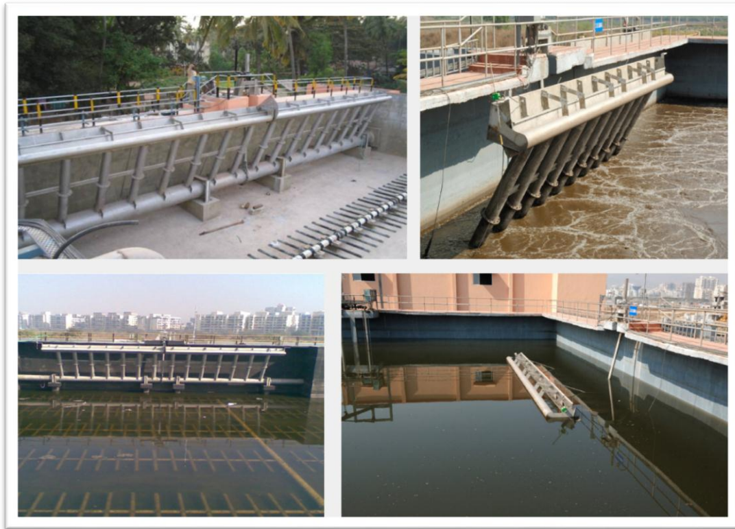
Figure 4: Sequencing Batch Reactor (17 MLD) at Puducherry
