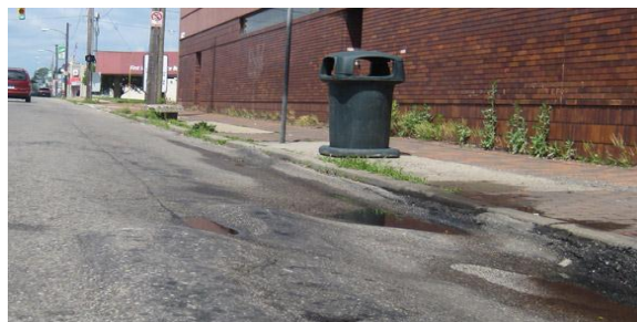
Fig-1: Shoulder failures on pavement
