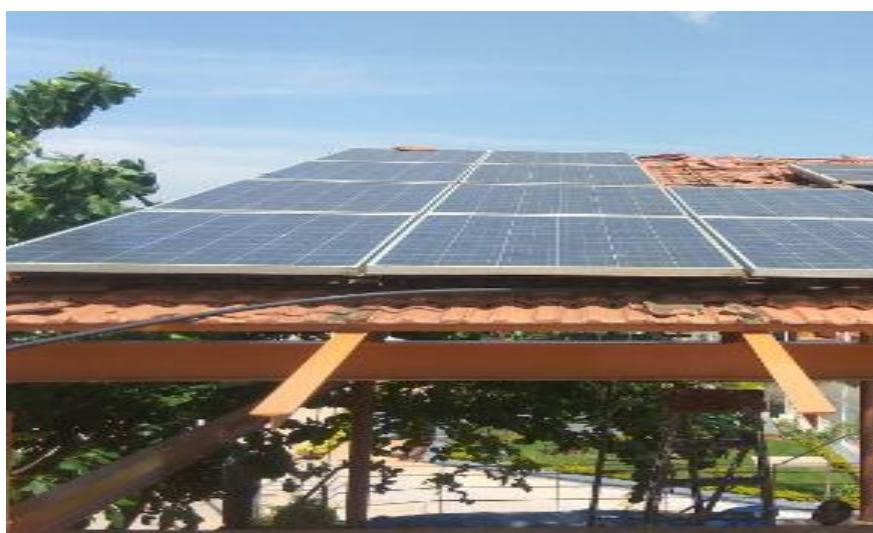
Figure 3: Solar PV Panels on the roof
