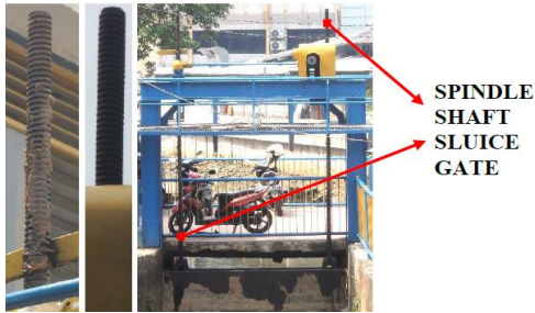
(H) Spindle Shaft Sluice Gate
