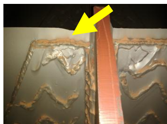
Figure 9. The tip and the edges of the impeller blades were wearing out very fast
