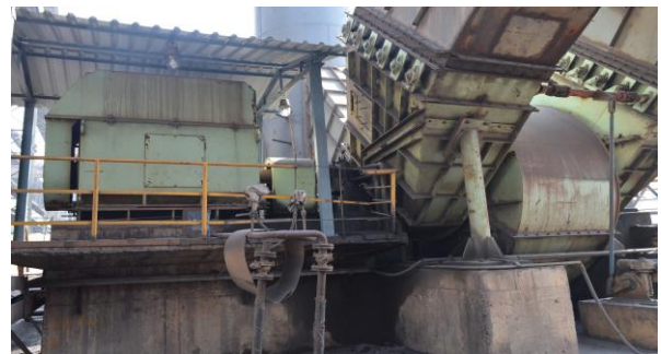
Figure 1. Picture of the ID Fan for the Blast Furnace Stock House
