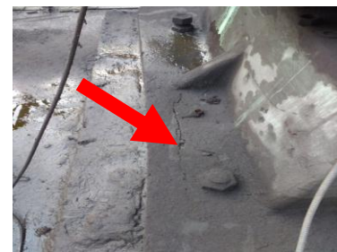
Figure 11. Initiation of Crack Propagation at the Base
