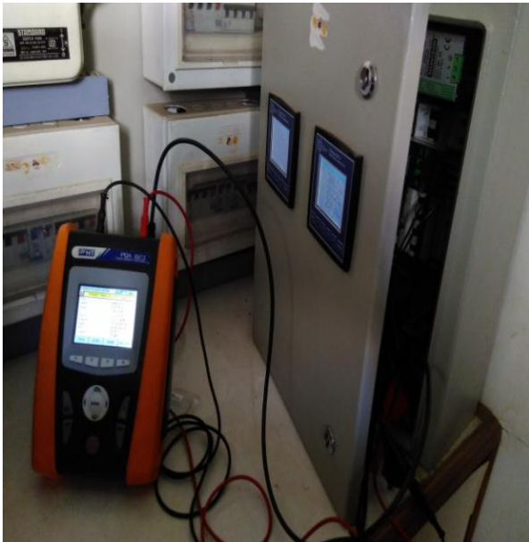
Figure 5: Internal connection of PQ analyzer connected to PV system
