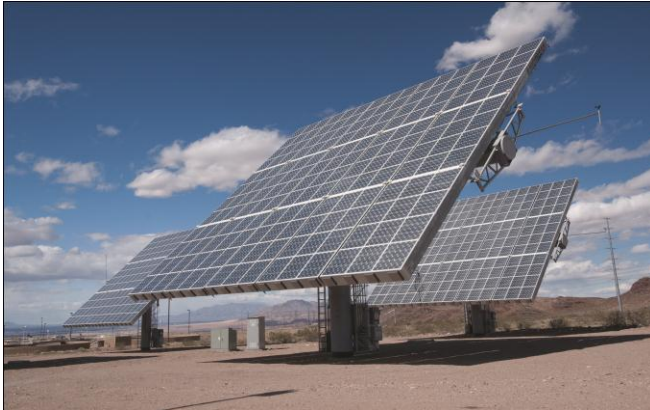
Figure 2. CPV project installed by Amonix in River Mountains WTF USA
