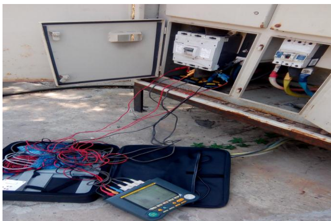
Figure 11. Connection of power quality analyzer
