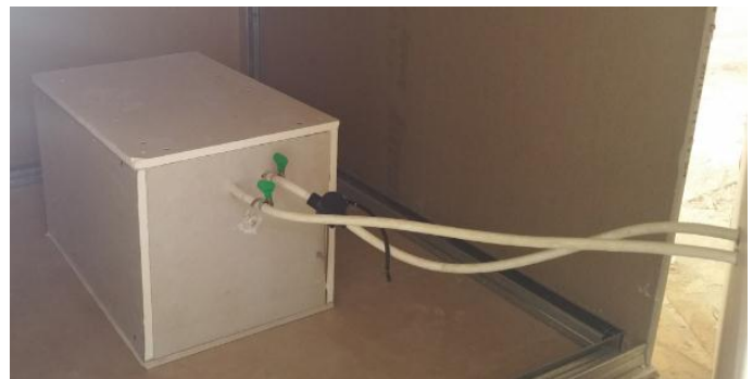
Figure 7 Piping for Air conditioning system
