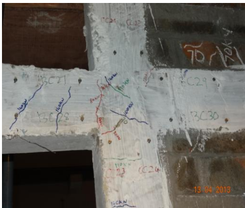
Fig.8 (b) Cracks at the joints
