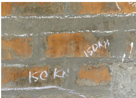
Fig.9. Occurrence of cracks in brick layers
