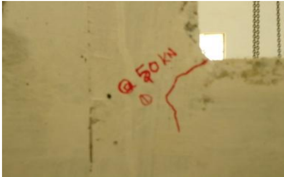
Fig.8 (a) Initial crack at the joints
