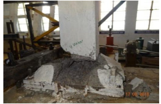
Fig.10. Final failure of frame
